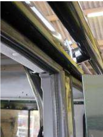
Finally mark, drill and bolt the B-pillar hoop through the second row floor.
